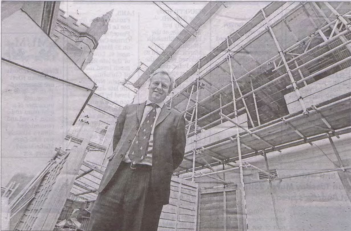
Elizabeth College principal George Hartley and the extension work that has started on the new maths block. The improvements will cost in the region of £450,000. (Picture by Tom Tardif, 1379385)
